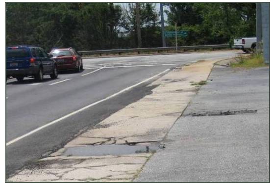
Sidewalk disrepair along Fleetwood Avenue near SC intersection
